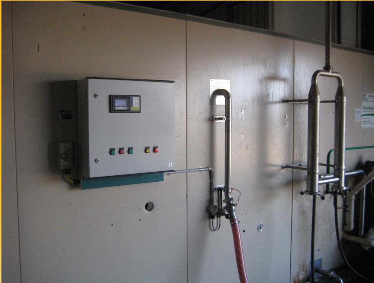
Green Cleaning unit controller in Horfield, Northern Victoria. Designed and built by GEA Farm Technologies. Chemicals supplied by Tasman Chemicals
