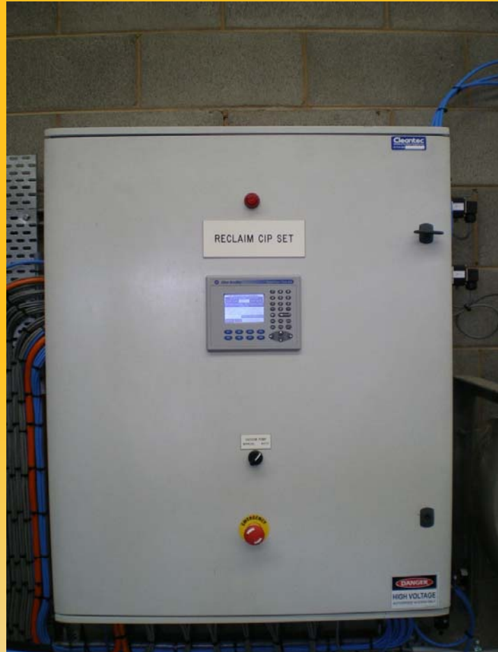
Controller for Green Cleaning system in Wangoom, Western Victoria. Designed and built by Cleantec – A division of EcoLab
