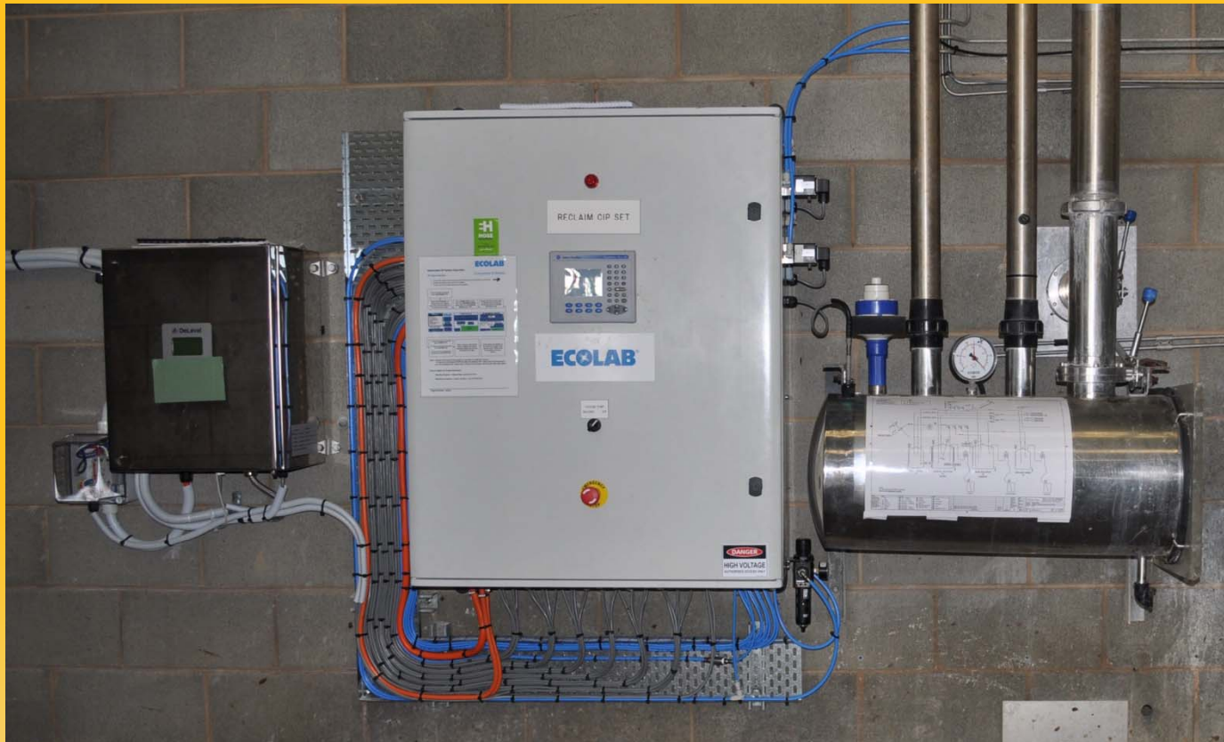
Controller for Green Cleaning system in Wangoom, Western Victoria. Chemicals supplied, system designed and built by Cleantec – A division of EcoLab.
